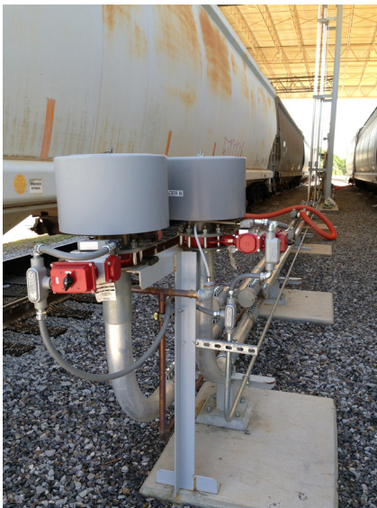
Typical Air Manifold
