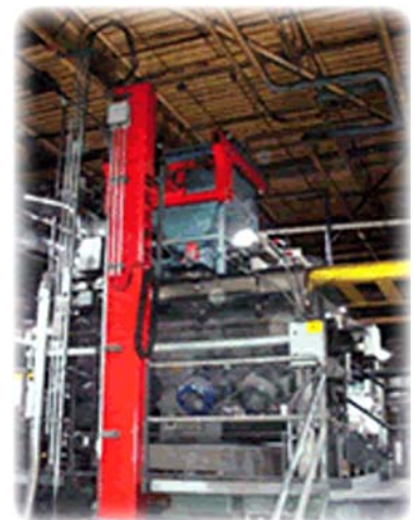
IBC docked atop the mixer, discharging product
