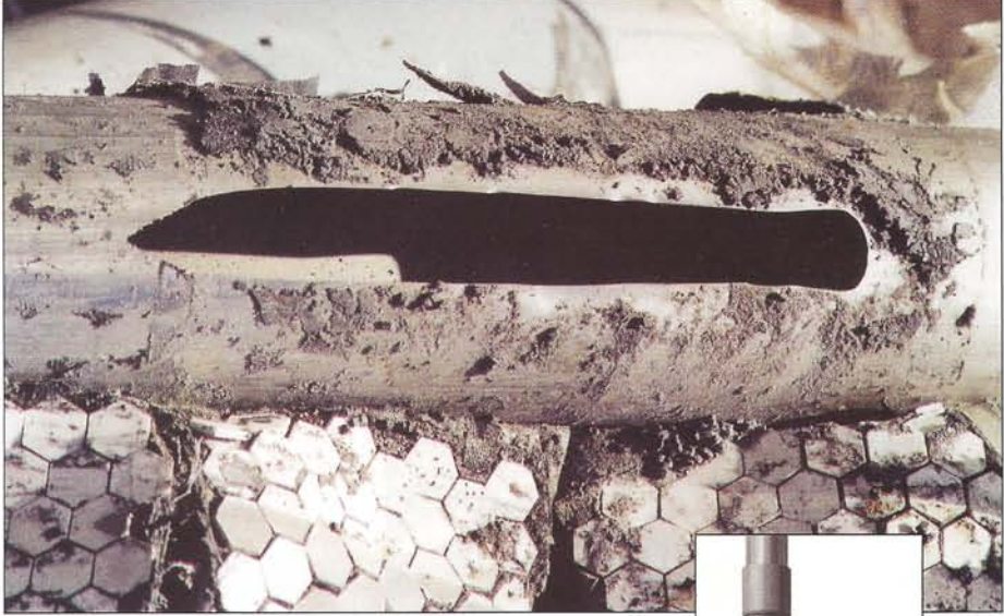
A common sight at RheTech before the HammerTek Smart Elbows® were installed was an attempt at patching with ceramic tiles and duct tape.
