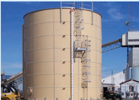
Bolted RTP - Process Liquids
