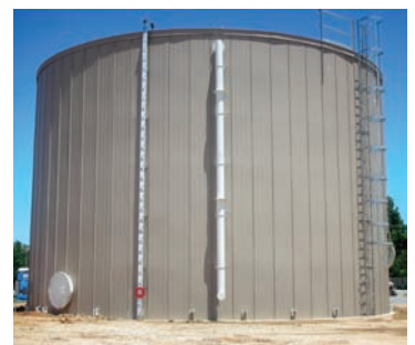
Fire Protection Tank
