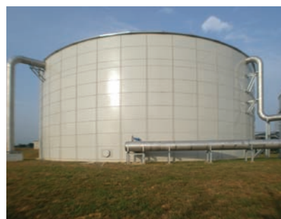
Potable Water Storage
