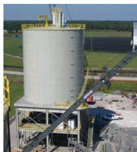
Bolted RTP - Process Storage
