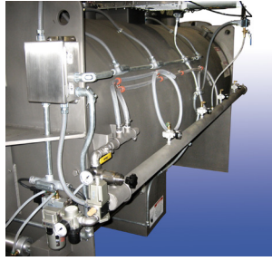
Compressed air header to seals and discharge valve and NEMA 4x SS J-Box for single phase components
