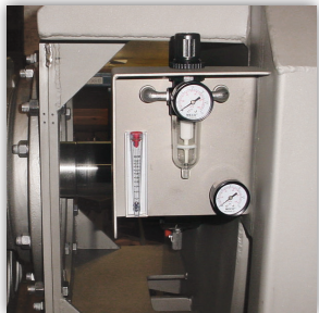
Air purged seals with flow meters
