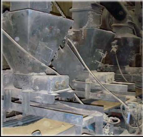
(3) Screw Feeders to feed 4 - 55 PPM Volumetric, Operator Monitoring Required
