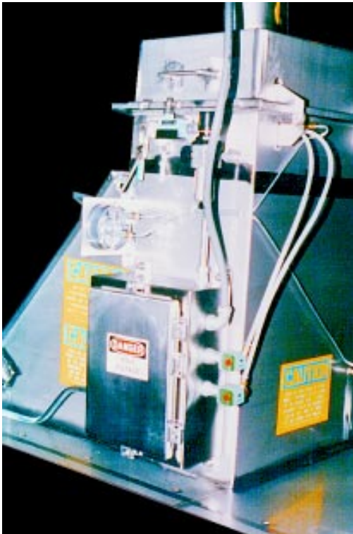
Waterproof electricals in stainless steel box; Magnehelic differential pressure gauge
